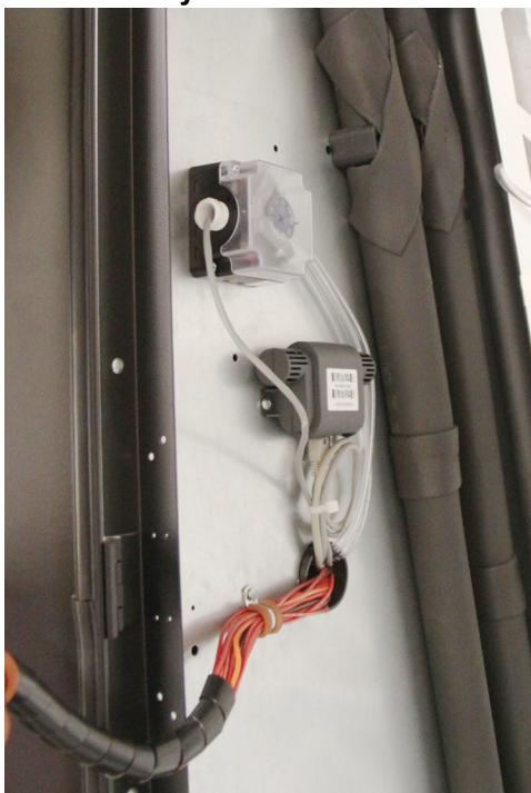
Figure 95 Return air temperature and humidity sensor viewed from the rear of the unit
